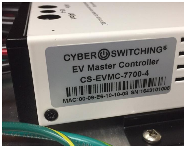
Figure 8: MAC and SN are listed on the side of the controller unit.
